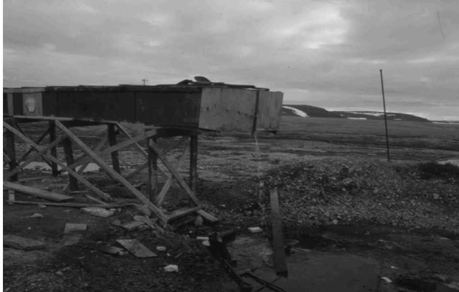
Figure 6. This utilidor, which was recently dismantled, is releasing sewage from the Resolute Bay (Cornwallis Island), North Base into a series of streams and ponds. The effluent ultimately reaches Meretta Lake, about 1.6 km downstream.
